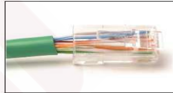
Bad Connector - Wires are untwisted for too great a length.
